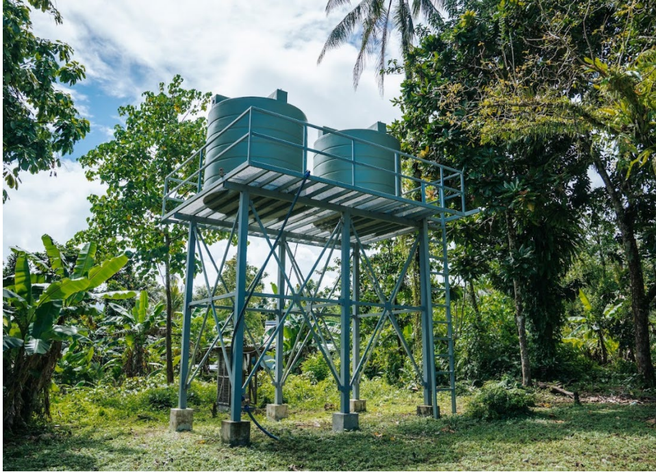
Caption: The two 10,000 litre water tanks in Qurasae are helping to provide 140 people clean and reliable running water for drinking and household use.
